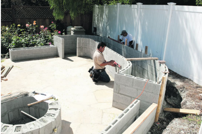
The Huffs' outdoor kitchen is still in the construction phase Photo Doug Kohen
